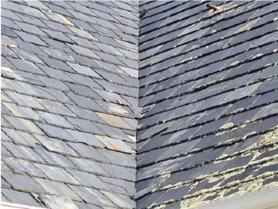
Ref # 4.2 - Some dislodged roof slates in the valleys.
