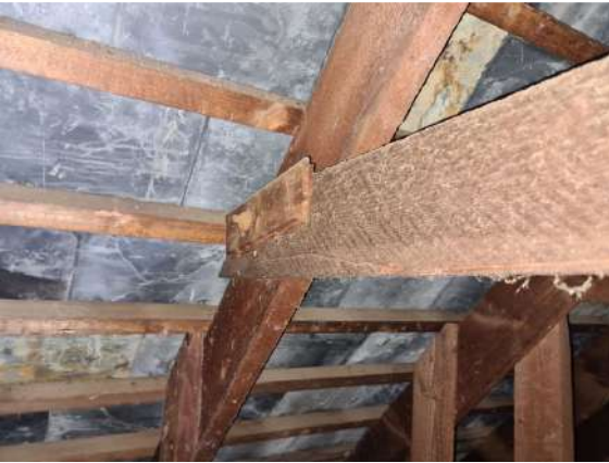
Ref # 5.1 - Minor cracks in some roof timber joists.
