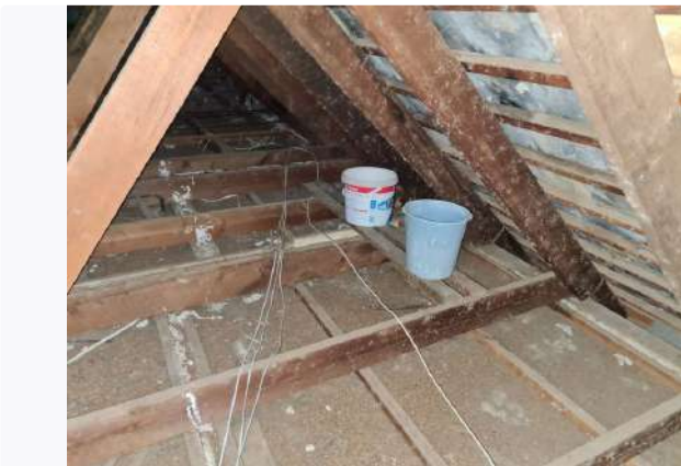
Ref # 4.1 - Containers in the roof due to active or previous roof leaks.
