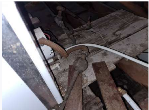
Ref # 6.2 - No isolator installed.
