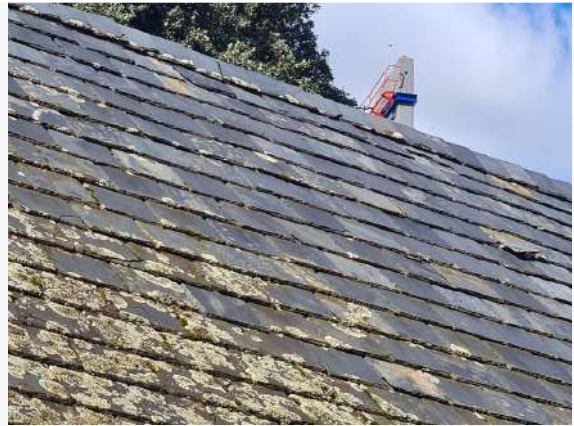
Ref # 4.1 - Moss growth on some areas of the roof covering.
