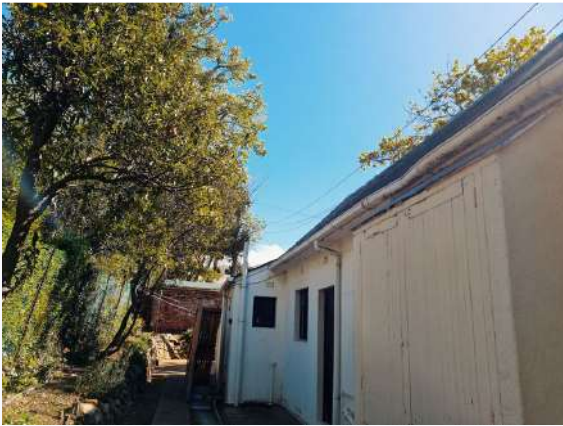
Ref # 4.3 - Gutters sagging in places and filled with debris.
