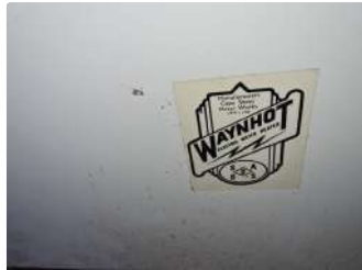
Ref #6 - Electric Geyser with tank
