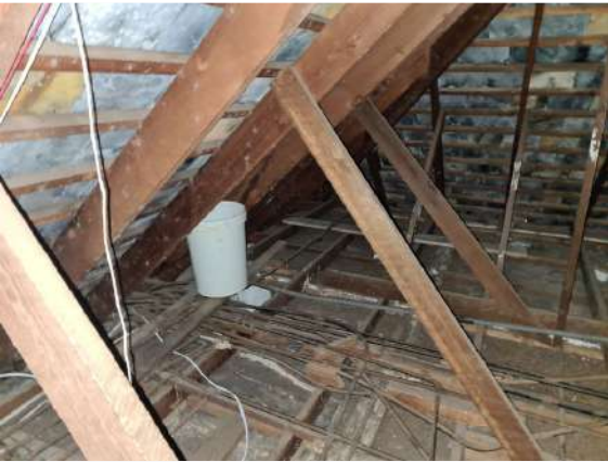
Ref # 4.1 - Containers in the roof due to active or previous roof leaks.
