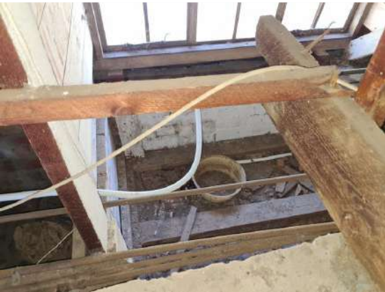
Ref # 4.1 - Containers in the roof due to active or previous roof leaks.
