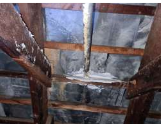
Ref #4 - Sealing of the roof covering around piping due to water penetration.
