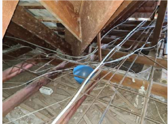
Ref # 4.1 - Containers in the roof due to active or previous roof leaks.
