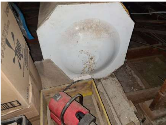
Ref # 6.1 - No drip tray installed.
