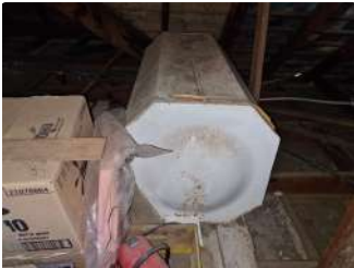
Ref #6 - Electric Geyser with tank
