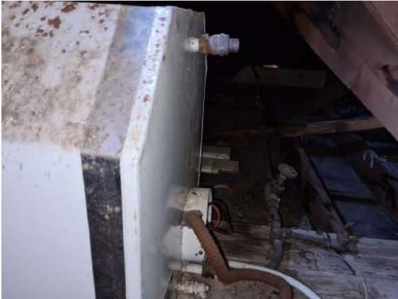
Ref # 6.3 - Thermostat cover plate not fitted / loose.
