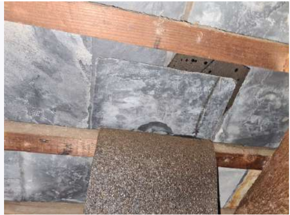
Ref # 4.1 - Some roof slates loose, cracked , damaged or dislodged.
