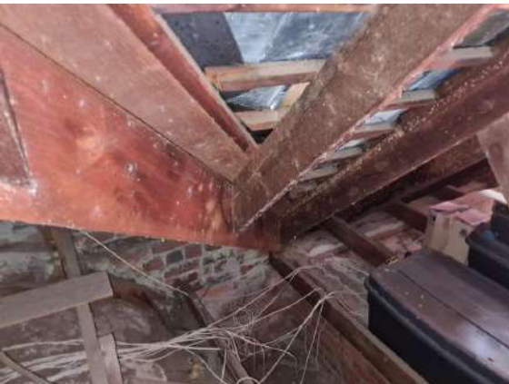
Ref # 5.1 - Minor cracks in some roof timber joists.
