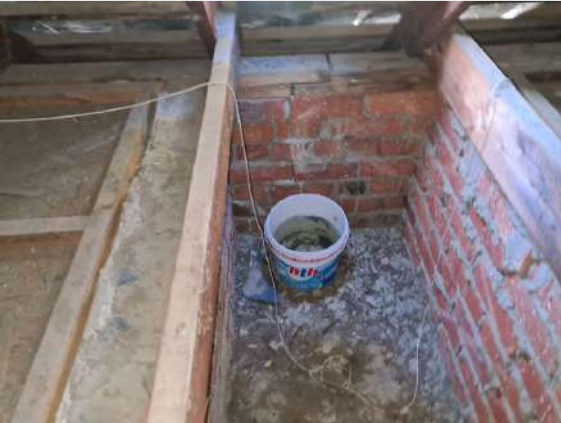
Ref # 4.1 - Containers in the roof due to active or previous roof leaks.
