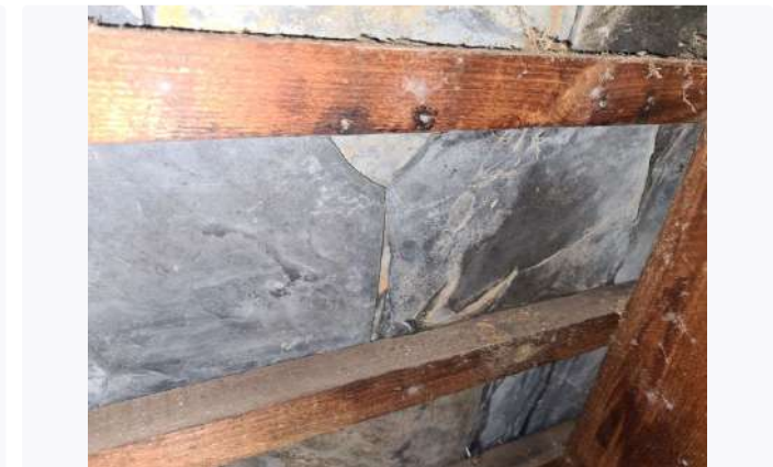
Ref # 4.1 - Some roof slates loose, cracked, damaged or dislodged.
