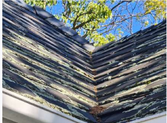
Ref # 4.2 - Valleys filled with debris.
