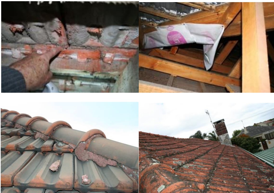
Moisture ingress over the years has resulted in soft and fungus-invested roof battens (top left); plastic nailed under the roof valley in a vain attempt to stop a leak (top right); cracked and dislodged mortar bedding of ridge tiles (bottom left); old roof with a noticeable sag (bottom right).
