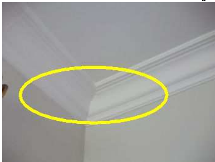
Dining room south west corner - movement cracks in cornice
