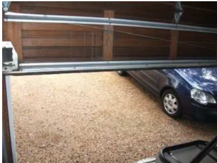
Double garage door operational
