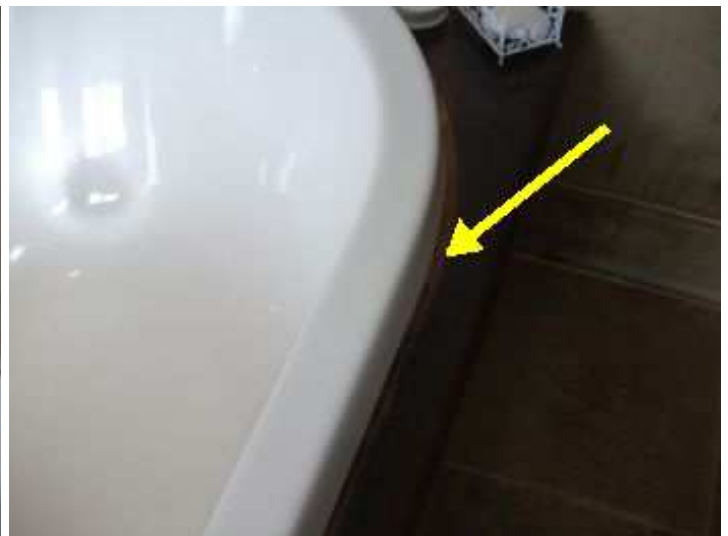
Main en-suite bathroom - movement between bath and enclosure visible
