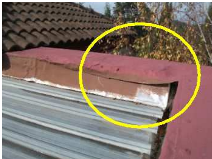
Entrance hall roof south west corner - untidy waterproofing / flashing
