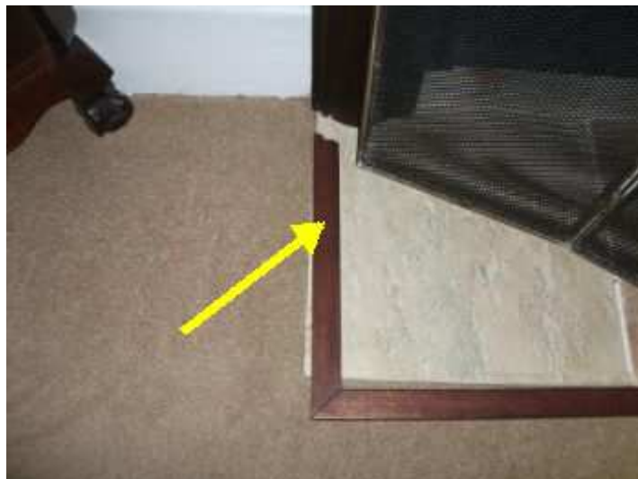
Dining room - fireplace hearth timber surround loose
