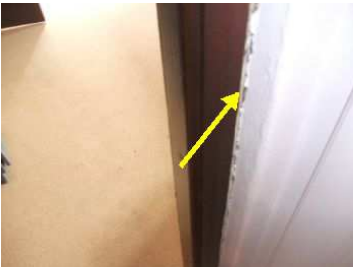
Bedroom 1 - minor door frame movement resulted in cracked plaster
