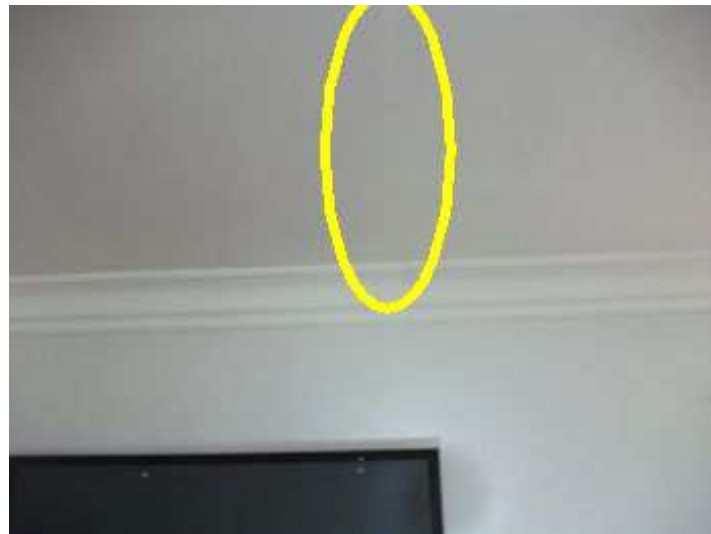
Family room north wall - movement crack in ceiling structure
