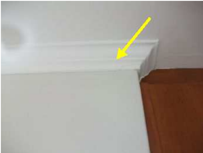
Main bedroom - movement cracks in cornice
