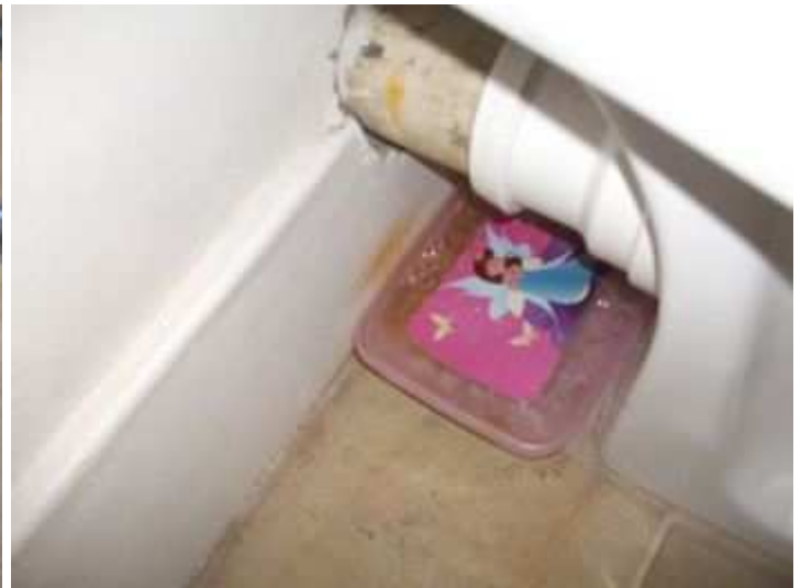
Bedroom 1 en-suite bathroom - possible leak at toilet waste pipe
