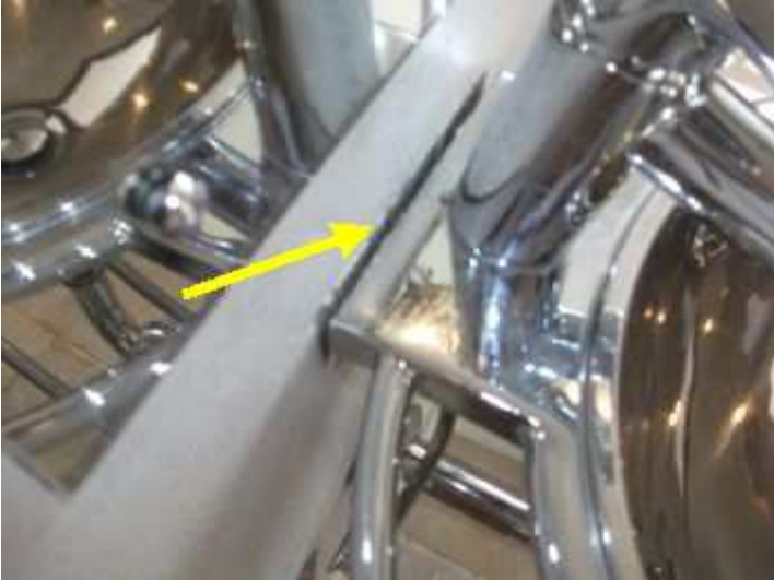
Bedroom 1 en-suite bathroom - basin loose
