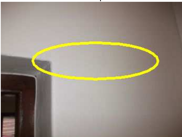
First floor lounge door - movement or settlement crack at door head
