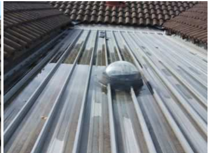
Entrance hall - standing water on roof sheets
