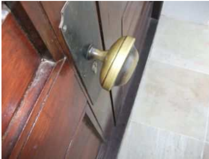
Front door - loose door knob - externally and internally
