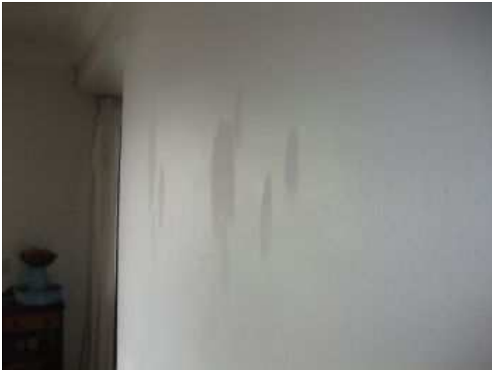
Family room south wall - repair marks on wall
