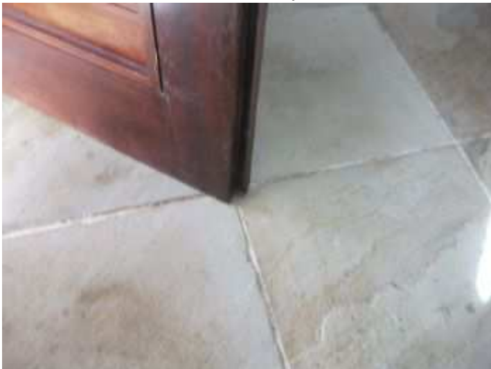
Family room - door catching on floor tiles
