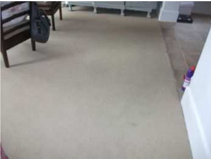
Main bedroom - carpets with general wear and tear marks
