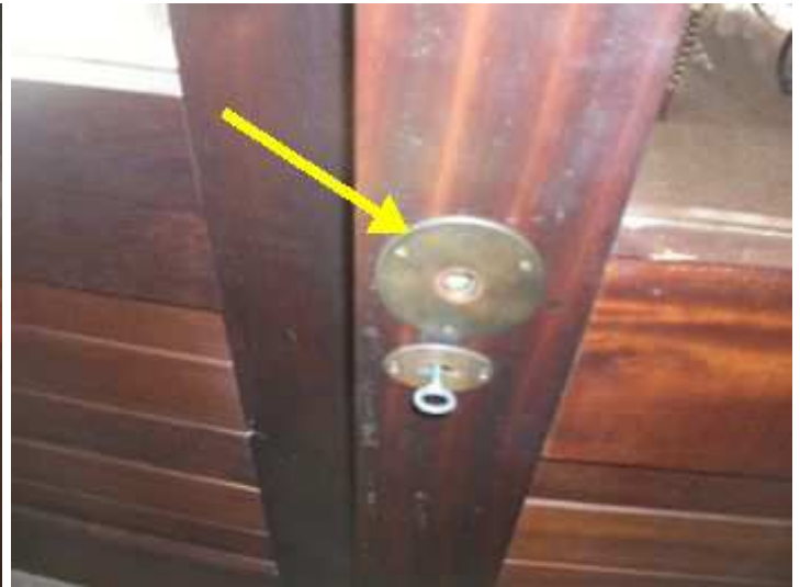
Family room - door knob removed
