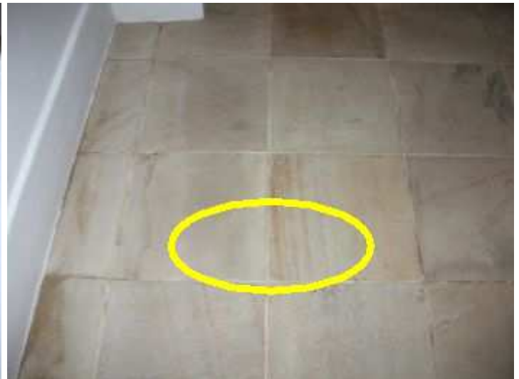
First floor passage (at main bedroom door) - cracked floor tiles
