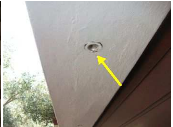
Garage door - rusted down lights
