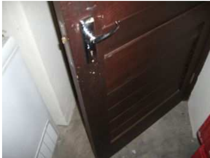
First floor lounge to garage - no fire door installed - does not comply with regulations
