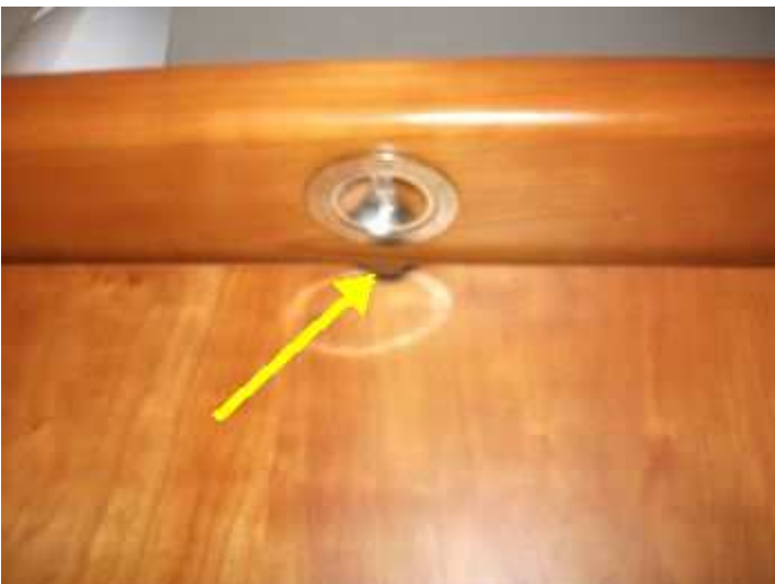
Kitchen south wall - burn mark on door caused by heat from down lighter
