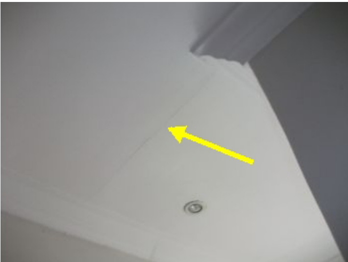
Bedroom 1 en-suite bathroom - movement crack between ceiling boards
