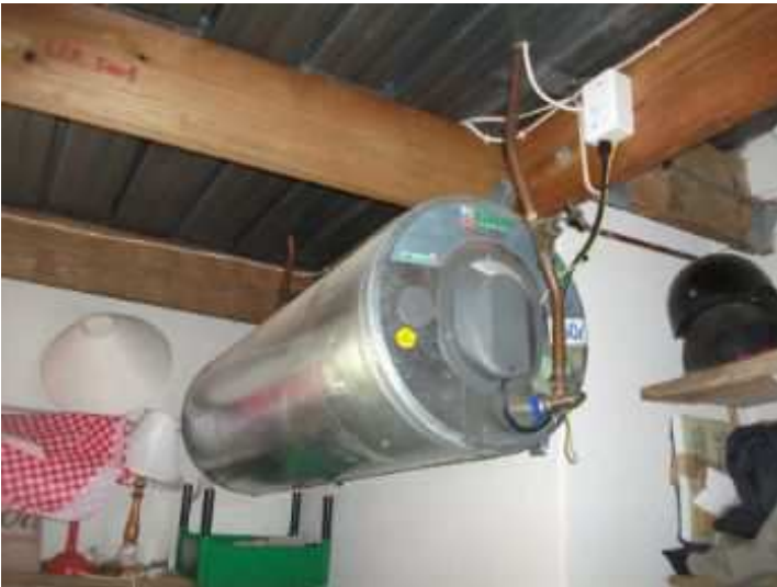
Geyser installation in garage
