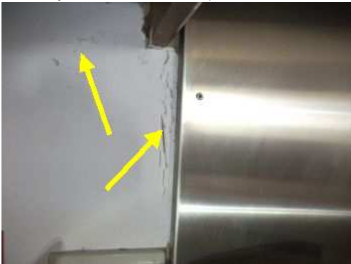
Kitchen west wall - flaking paint next to stove splashback
