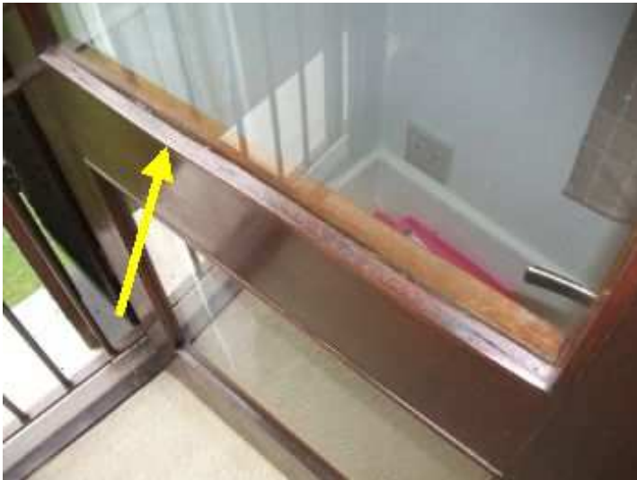
Main bedroom - cracked and warped glazing timber strip
