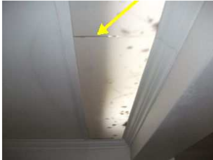
Entrance hall - skylight dirty - movement between panels
