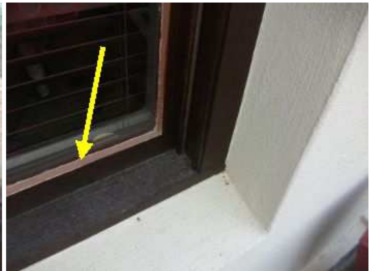
First floor lounge - some window panes with new glazing putty - should be varnished to prevent putty from drying out
