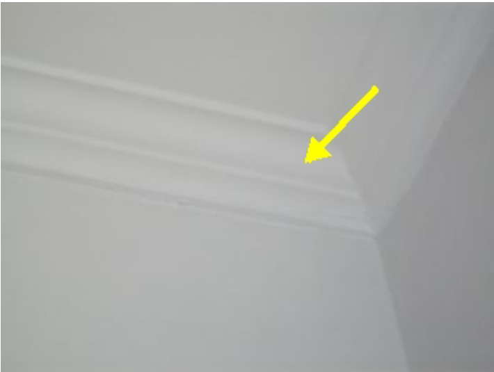
Bedroom 1 - movement cracks in cornices
