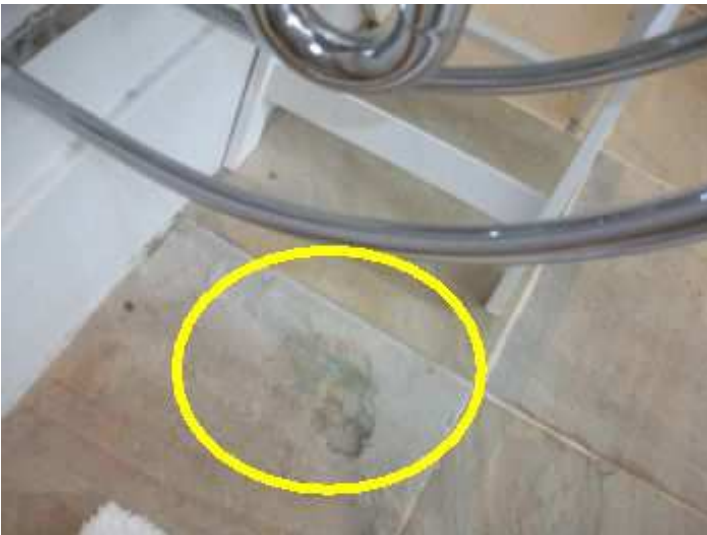
Bedroom 1 en-suite bathroom - water drip marks below basin waste pipe
