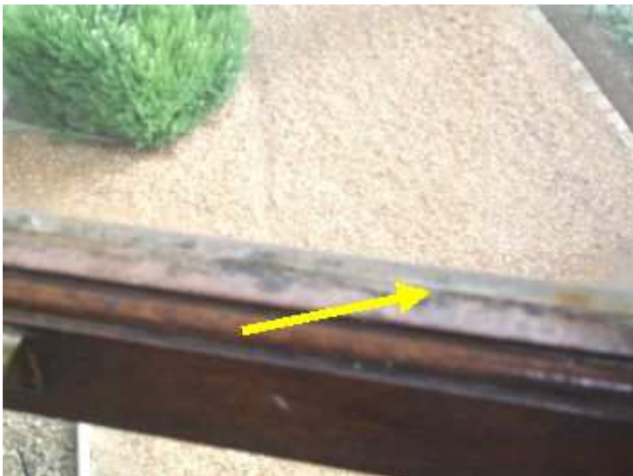
General comment - water ingress between frame and glass at some windows
