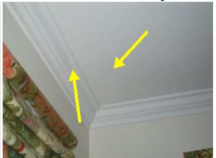
Study south west corner - movement cracks in ceiling and cornice
