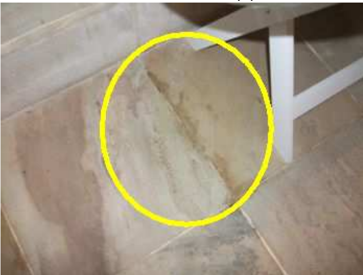
Bedroom 2 en-suite bathroom - water mark below basin - waste pipe dry at inspection
