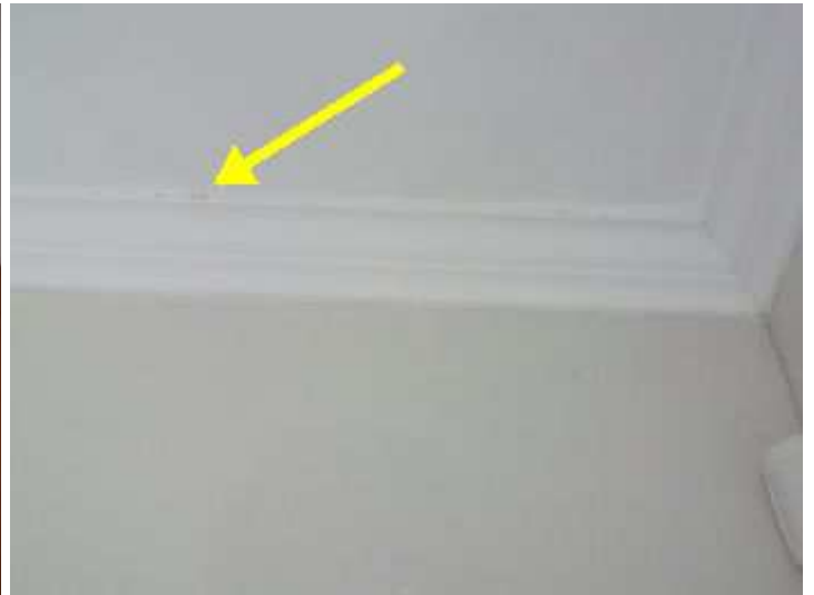
Main bedroom north east corner - movement cracks between cornice and ceiling boards
