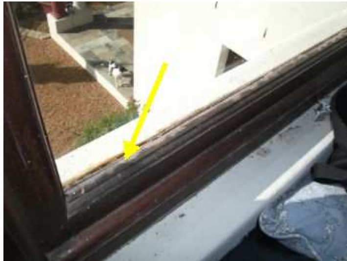
Garage - water ingress between glass and frame as a result of dry glazing putty
