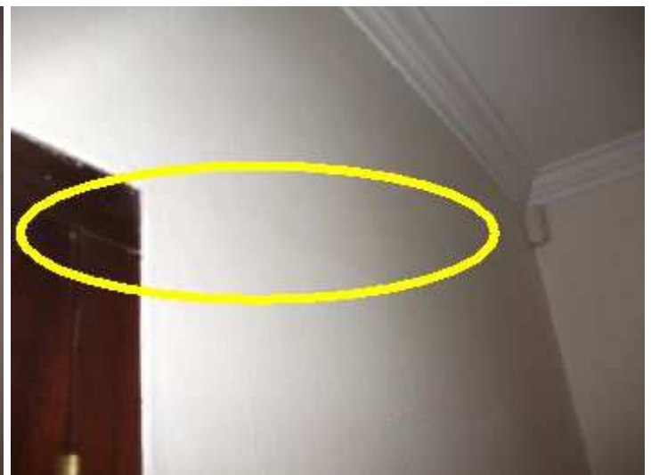
Study north wall - movement or settlement crack at door head
