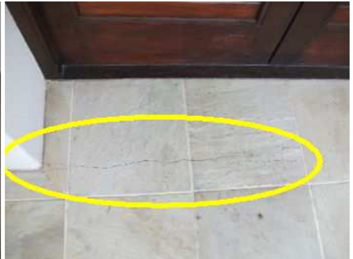
Front door - settlement crack at front door
