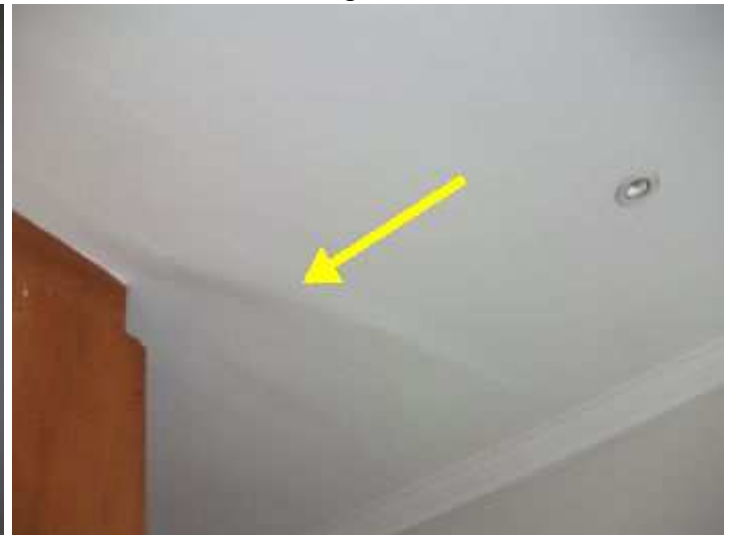
Main bedroom (between dressing area and bedroom) - movement crack between ceiling boards
