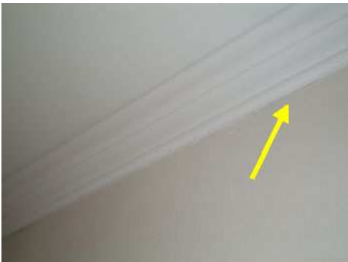
First floor lounge west wall - movement cracks between cornice and wall
