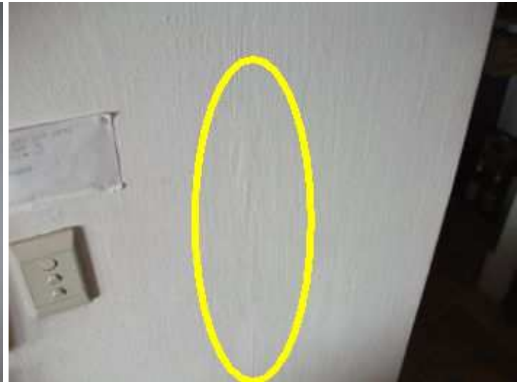
Kitchen to wine cellar - repaired crack visible
