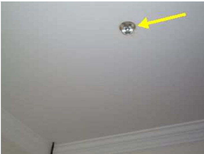
First floor lounge - down light fitting shell missing
