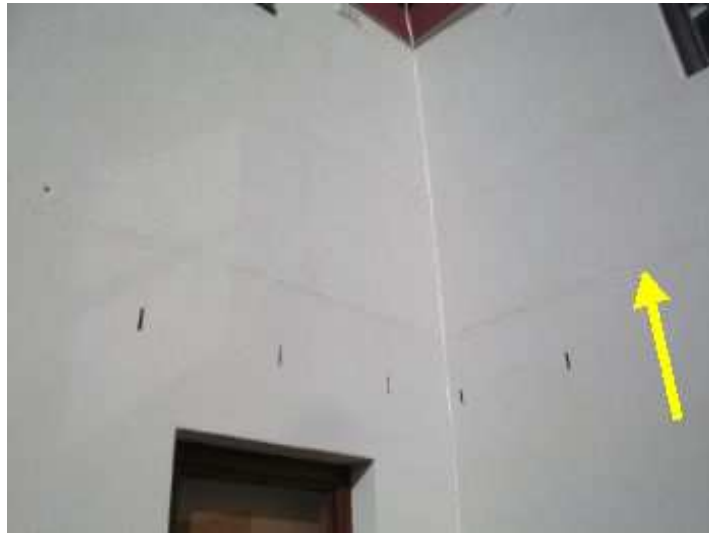
Guest bedroom east facing wall - possible water ingress at control joint caused damp internally - walls recently painted
