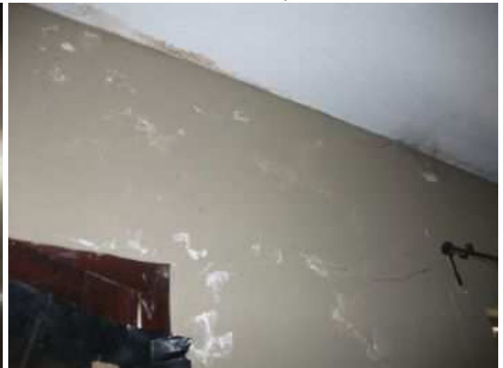
Guest bedroom east wall - penetrating damp
