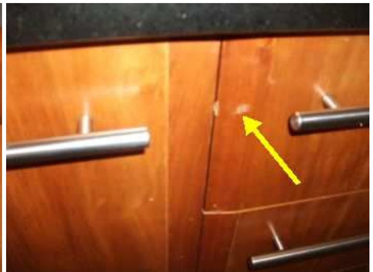
Kitchen - general wear and tear marks to some cupboards
