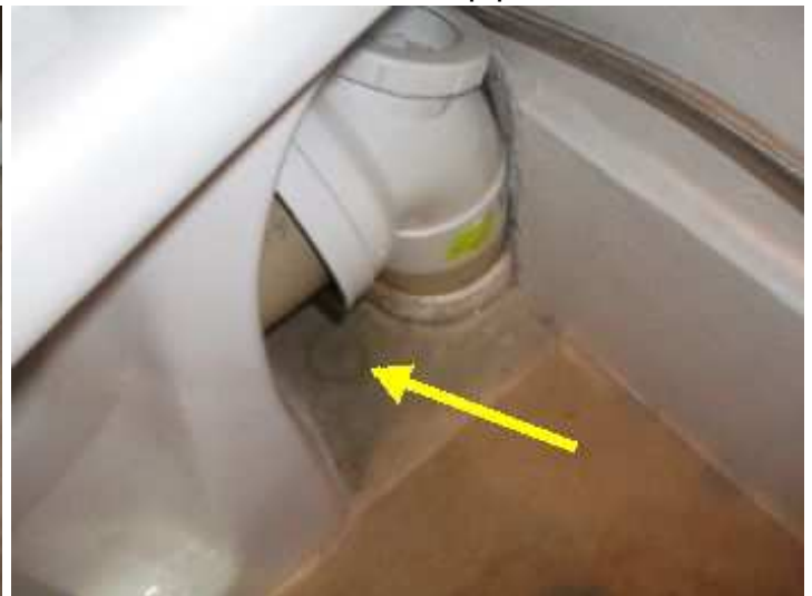
Bedroom 2 en-suite bathroom - leak at toilet waste pipe
