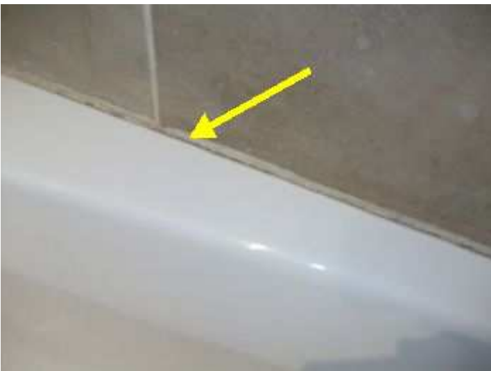
Bedroom 2 en-suite bathroom - bath not properly sealed at wall intersection
