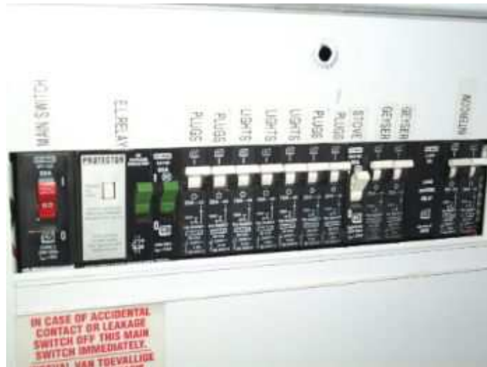
First floor lounge south wall - DB board in good condition
