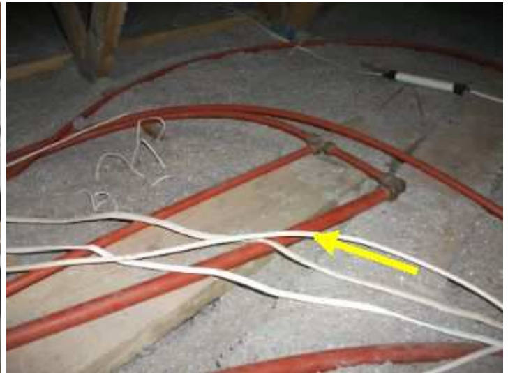
Geyser - hot water pipes should be copper or suitably rated (70 deg. C) plastic or composite pipe
