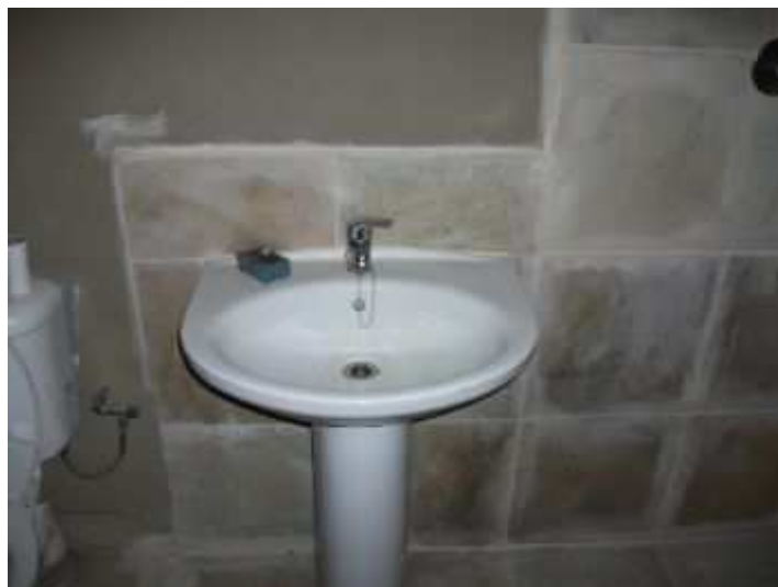
Guest bedroom en-suite bathroom - tile cleaning and painting not finished
