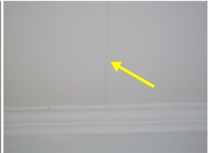
Bedroom 1 north wall - movement crack between ceiling boards
