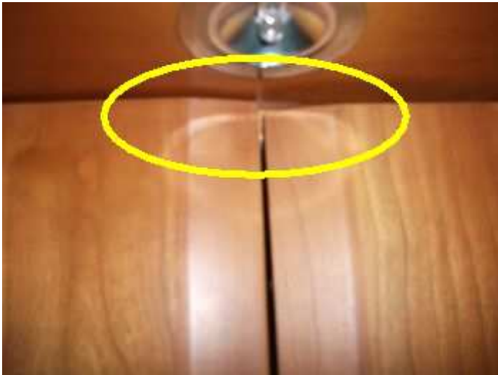
Kitchen - some cupboard doors should be realigned
